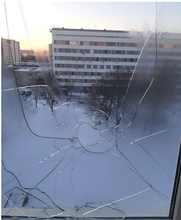
Figure 1. A view through the damaged window from the operative theatre
